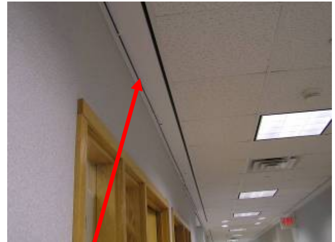
Cable feeding remote antennas
